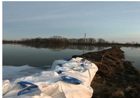
Figure 5: the ultimately implemented embankment did halt the piping process
