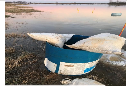
Figure 4: bags to ballast the barrels are not effective to achieve sealing and avoid leakage
