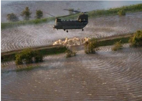
Figure 2: Deployment of Chinook helicopter in dike breach Wainfleet, 2019
